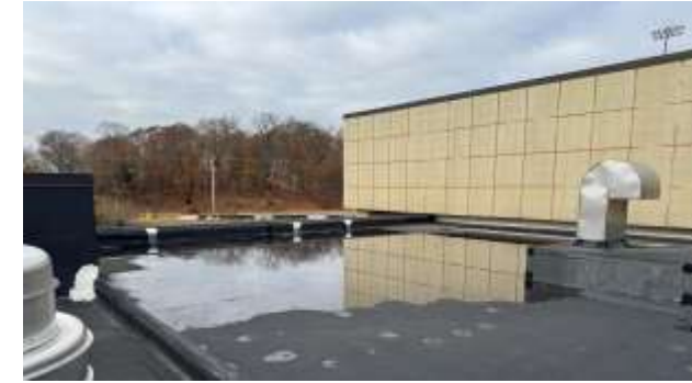
Significant Ponding on Roof Membrane
