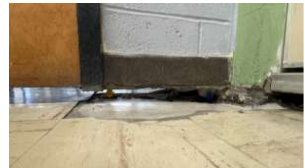
Slab Settlement in Wing C
