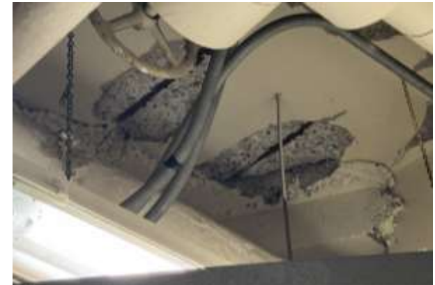
Exposed Rebar Below Pool Deck
